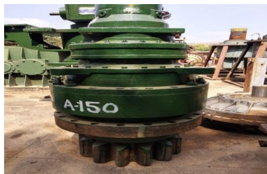
Fig:1 Mobile transfer conveyor 12/13 slewing gearbox
