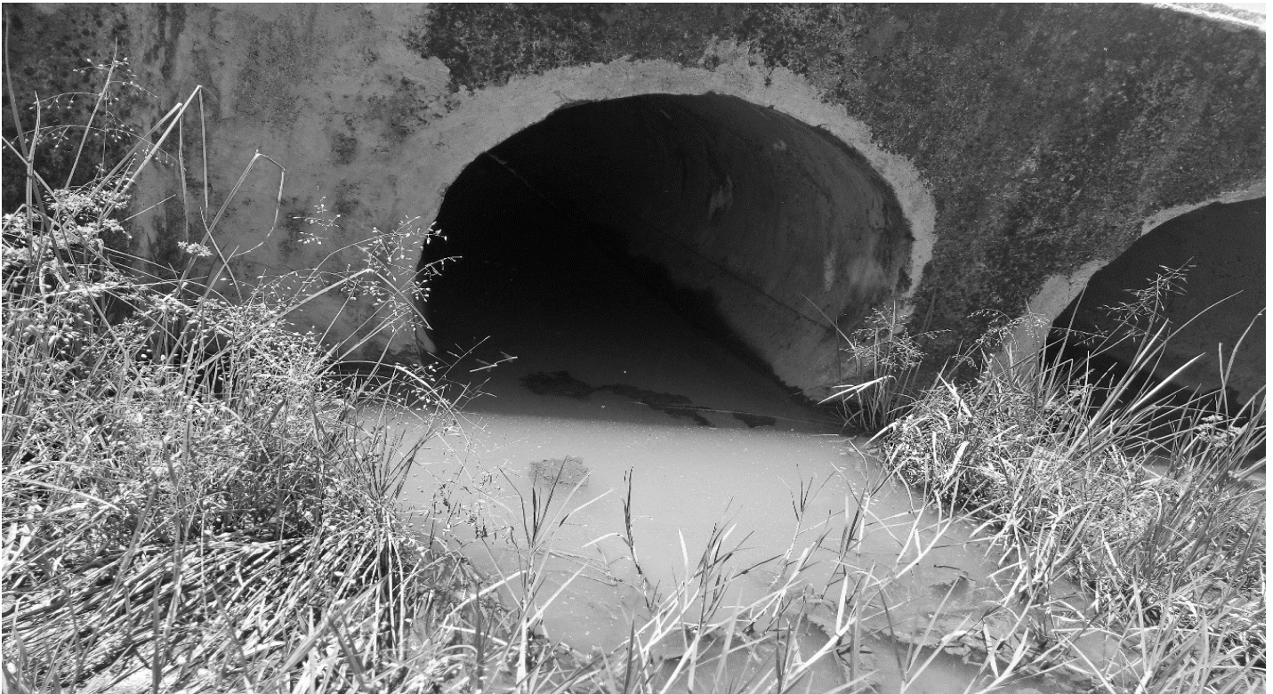
Plate 1.0: Picture of stagnant water under culvert at Lenana Estate in Narok Town Ward.
