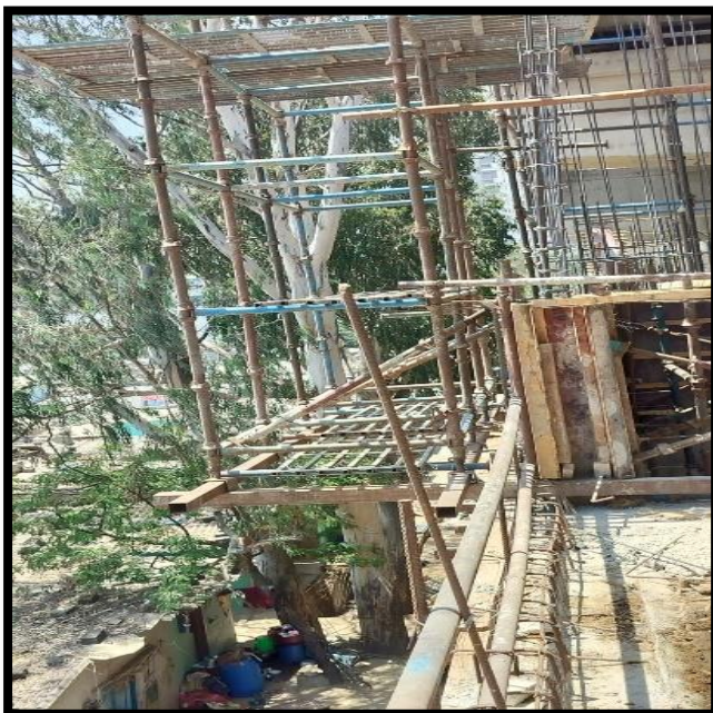
Overhead fall protection arrangements are not provided at adjacent to live road, materials may fall to the road.
