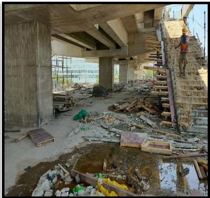
Poor housekeeping on site/Unwanted scrap and Debris observed on site creating tripping hazard. C & D waste not disposing regularly.
