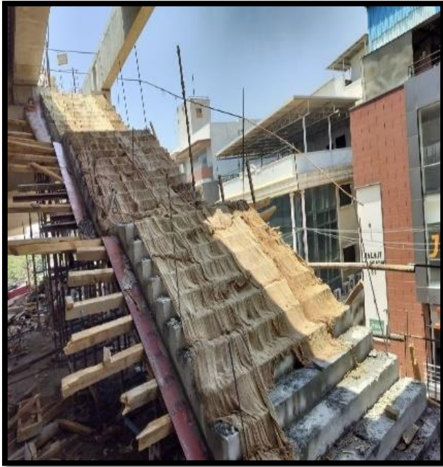
Workmen accessing unsafely, guard rail and fall protection not available.
