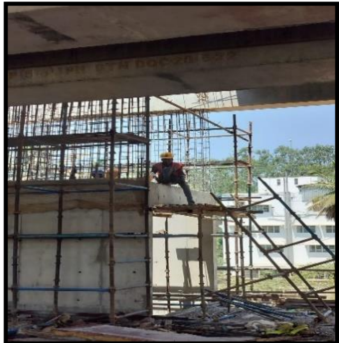
Workmen working at height without fall protection arrangements.
