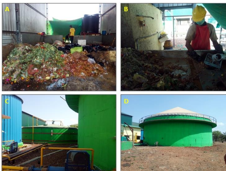
Fig. 16. A) Waste Collection Platform, B) Shredder-Mixer, C) UASB D) CSTR
