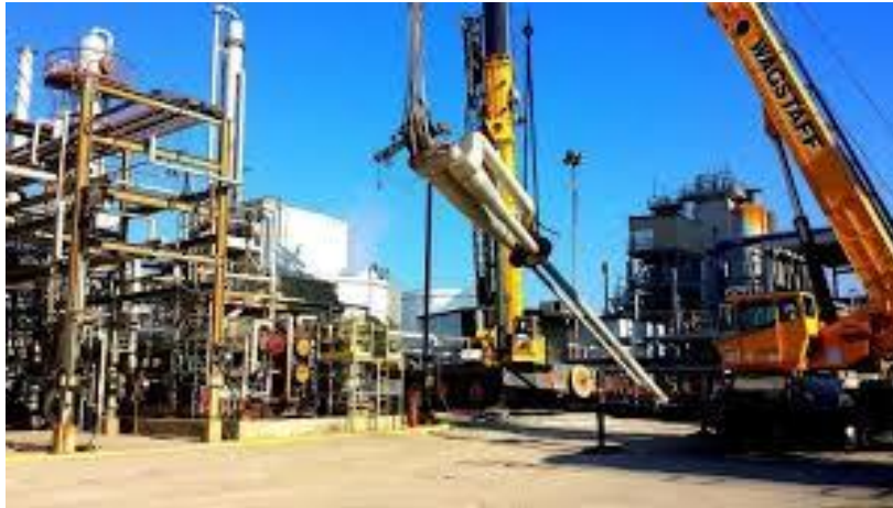
Fig. No. 25 Critical Lifting
