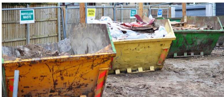
Fig. No. 20 Waste Segregation & Collection
