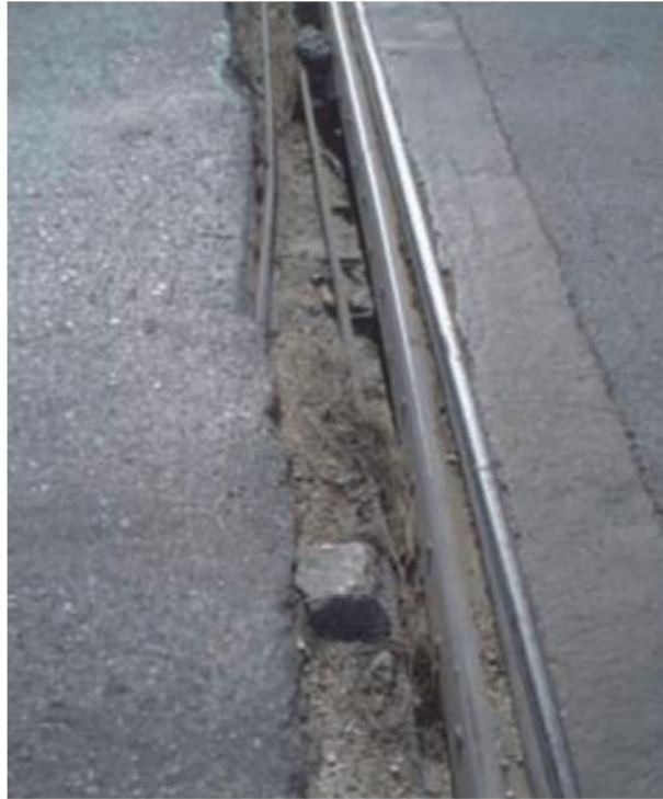
Figure 1.8. bridge concrete construction joint Cracked [9].
