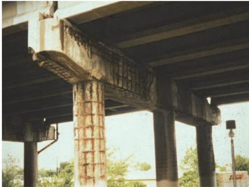
Figure 1.6. Cement reinforced metal piers with corrosion issues [7].
