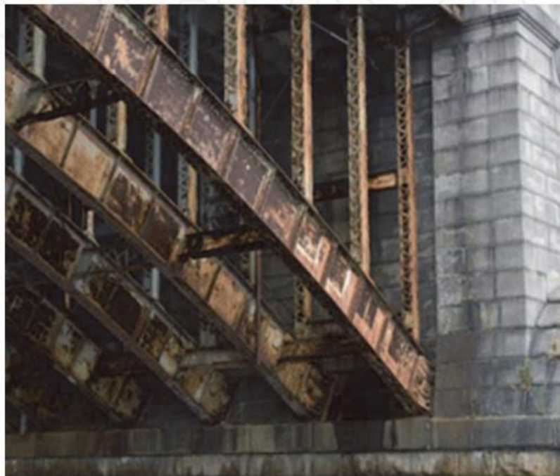
Figure 1.7. Corrosion issues on a structural steel bridge [8].
