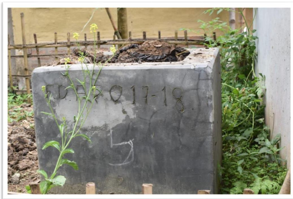
Fig 9: Slurry Inlet with loaded Biomass
