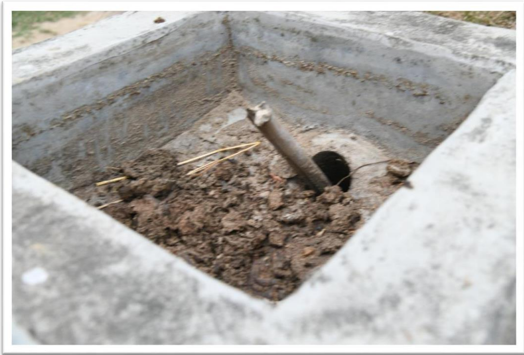
Fig 10: Slurry Inlet Tank at Sivasagar
