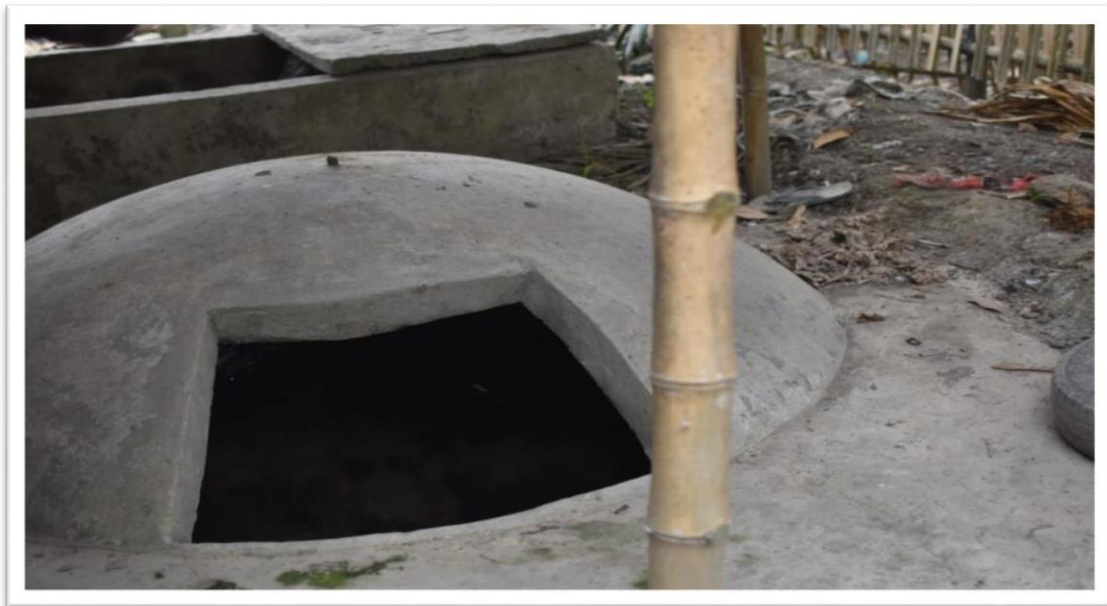
Fig 21: Digester converted into fishery tank due to manufacturing defect
