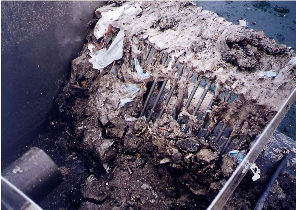
Fig. 3.2.1. Example of screenings collected on a manually cleaned rack. Note the gross material which includes pieces of paper and plastic wrapping. These can blind the screen unless regularly removed.
