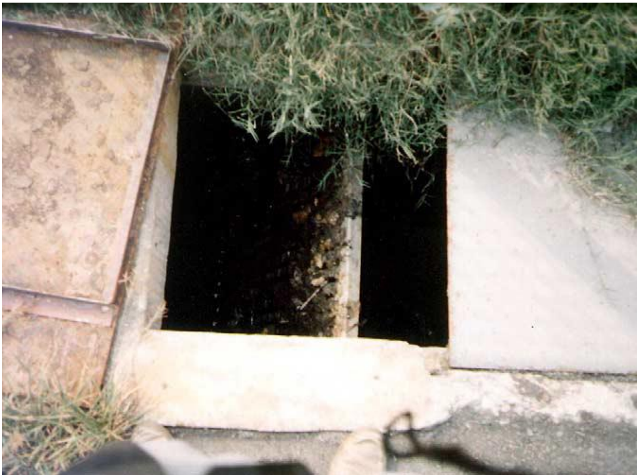
Fig. 4.2.2. Covered drain leading to the collection sump of an IWTP. The (removed) cover had been placed over a coarse screen. The easily removable covers facilitate the removal of screenings from the screen. The drain is shallow because the distance between the factory and IWTP is small.
