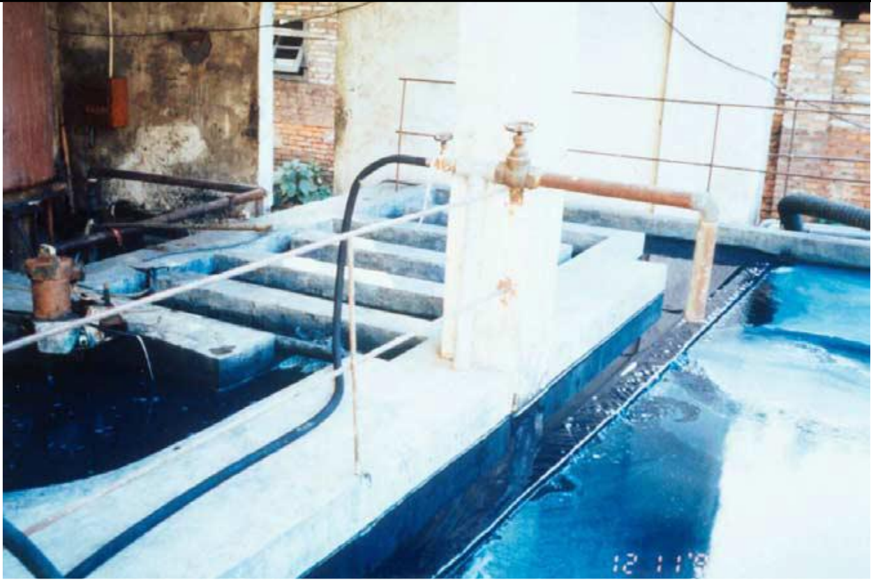
Fig. 4.4.3. Labyrinthine type flocculator (LHS) at a IWTP for a textile dyehouse. The dosing of the flocculant from a pipe just before the start of the first baffle of the flocculator can be seen on the LHS of the picture.
