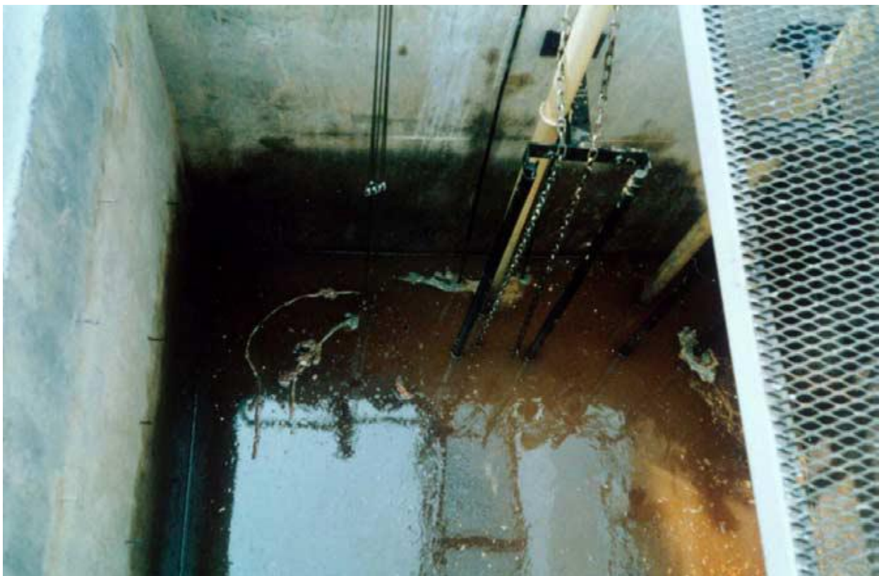
Fig. 4.2.1. Shallow wastewater collection sump at a personal care products factory. Submersibles are located in this sump to lift the wastewater to the next unit process in the IWTP. The sheen on the water surface suggests the presence of O&G.
