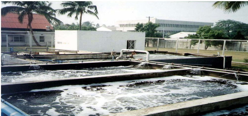
Fig. 3.4.1. Activated sludge plant for sewage treatment where the bioprocess is a combination of suspended and attached growth. The submerged biofilm support modules are located along a line running longitudinally and down the center of the tank.
