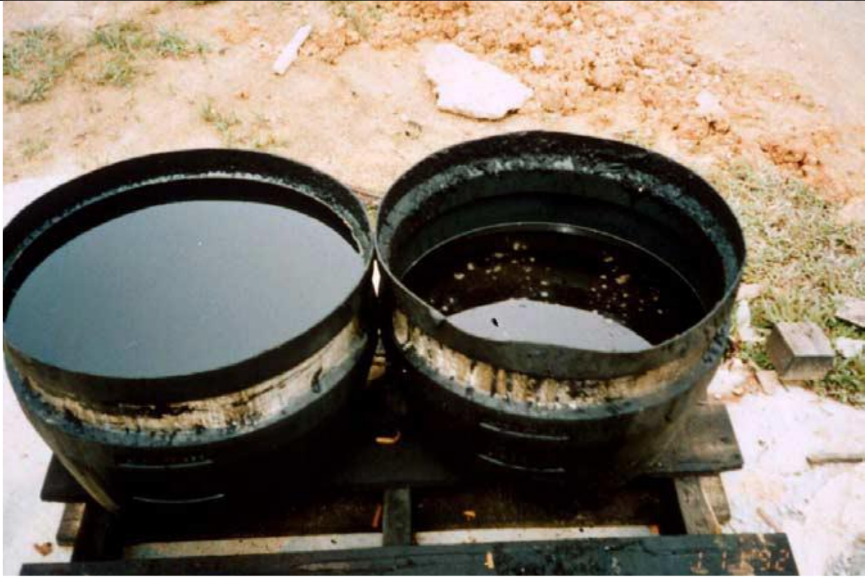
Fig. 4.2.5. Lubricating oil collected from the O&G trap at a soft drink bottling plant.
