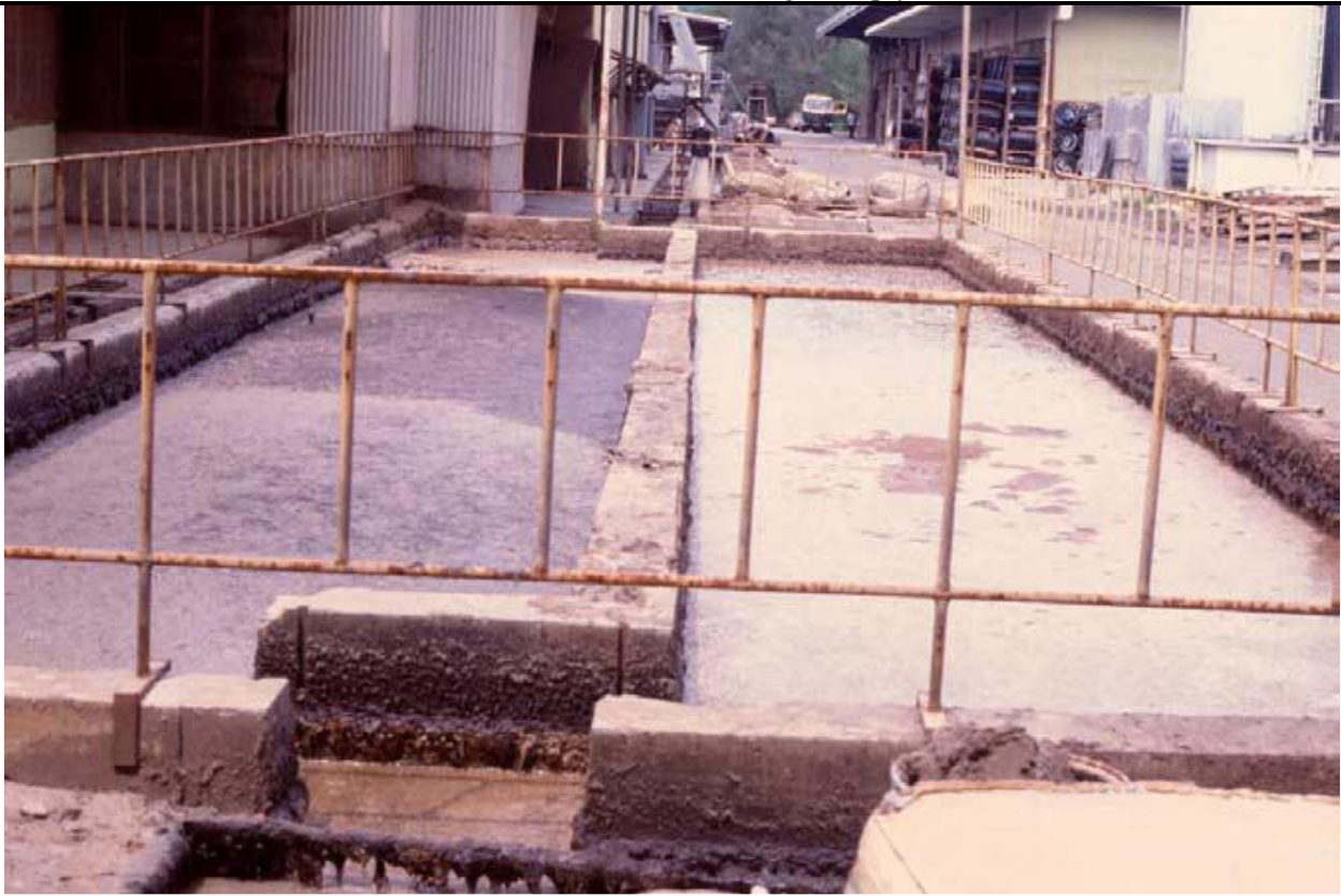
Fig. 4.3.1. Two-chambered aerated equalization tank at a lanolin extraction IWTP.
