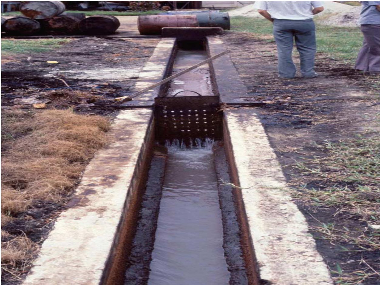
Fig. 4.2.3. Baffle plate O&G trap inserted into a surface drain leading to the IWTP at a palm oil refinery. The effectiveness of such a simple device may be seen from the O&G accumulated behind the baffle plate. While not reducing the wastewater’s O&G content to the required levels, the trap significantly reduced the O&G load which would otherwise be imposed on the next unit process.
