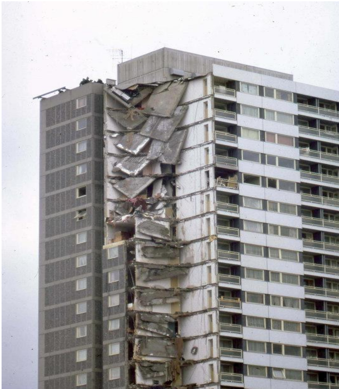
Figure 1.1 Ronan Point Incident
